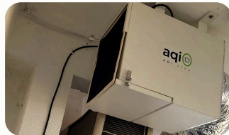
Ceiling hung above an AC outdoor unit
