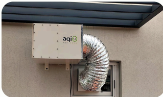
Wall mounted on a terrace
